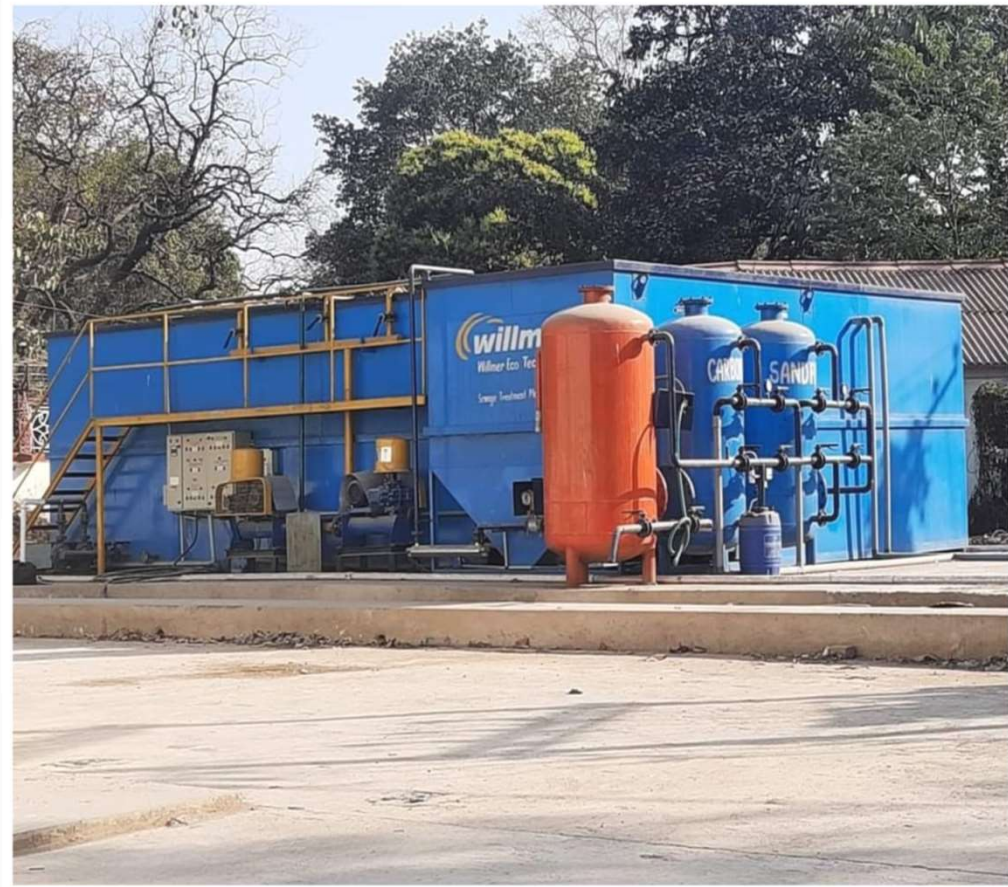
150 KLD STP Patna High Court, Bihar
