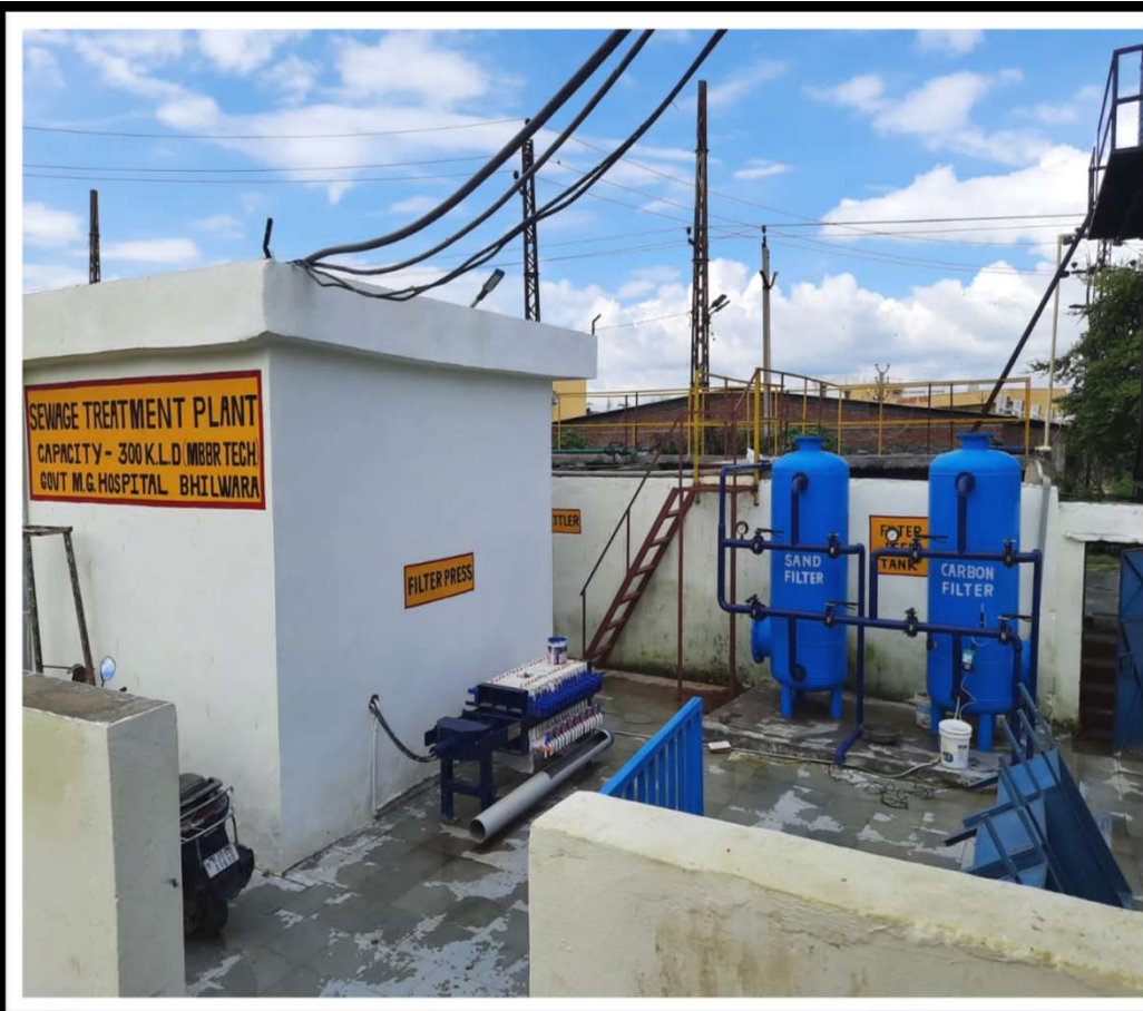
Mahatma Gandhi Hospital 300 Kld STP Bhilwara, Rajasthan
