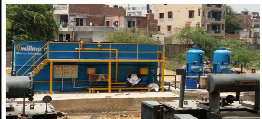
100 KLD S.T.P R.U.H.S, JAIPUR, RAJASTHAN
