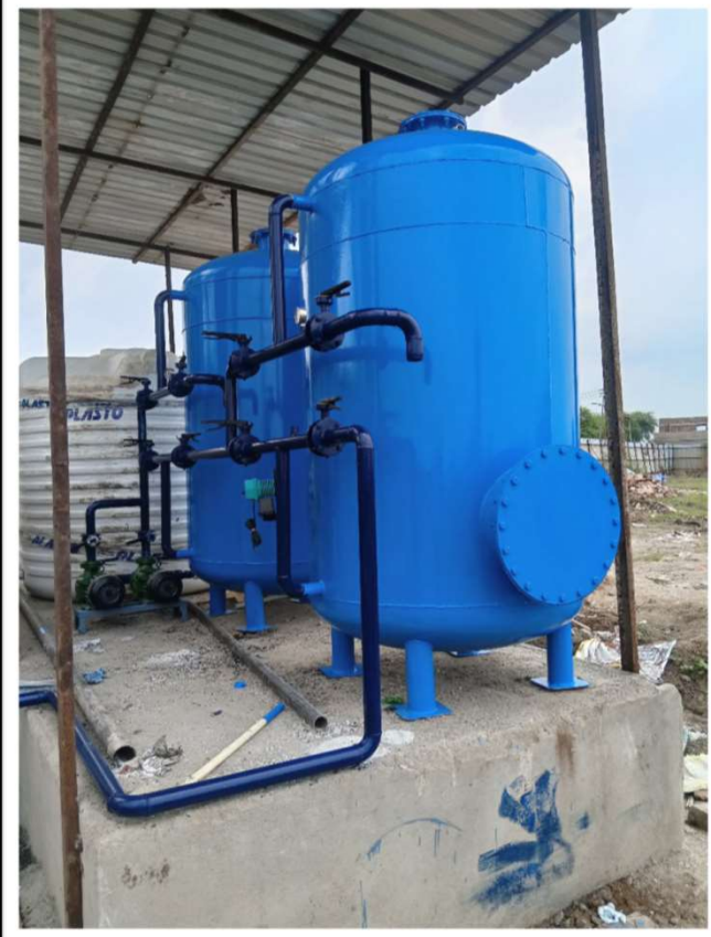
WATER TRETMENT PLANT Shubah Avenue & Shubah Sanskar KOTA RAJASTHAN
