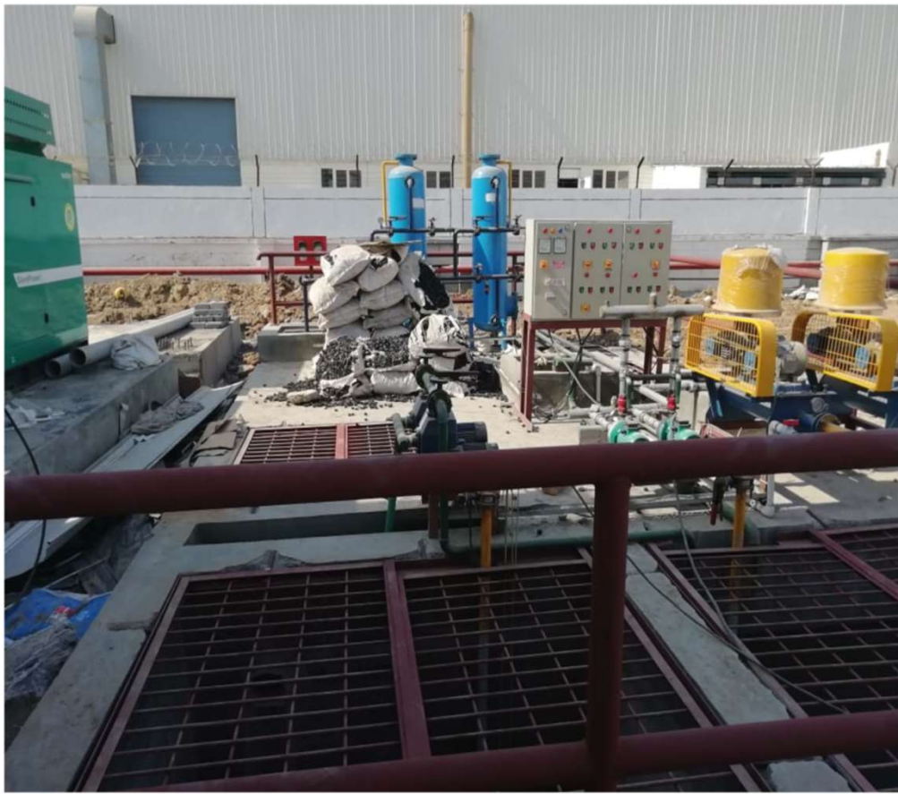
25 KLD STP Napino Auto and Electronics Limited, Halol, Vadodara, Gujrat
