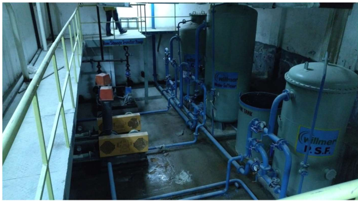
The Great Mall Of Kota, (Ahaluwalia Contract India Ltd.) 200 KLD STP
