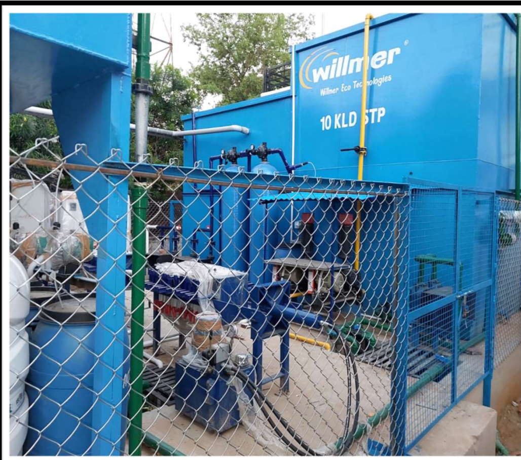
Pollution Control Board 10 Kld STP Pollution Control Board, Jaipur
