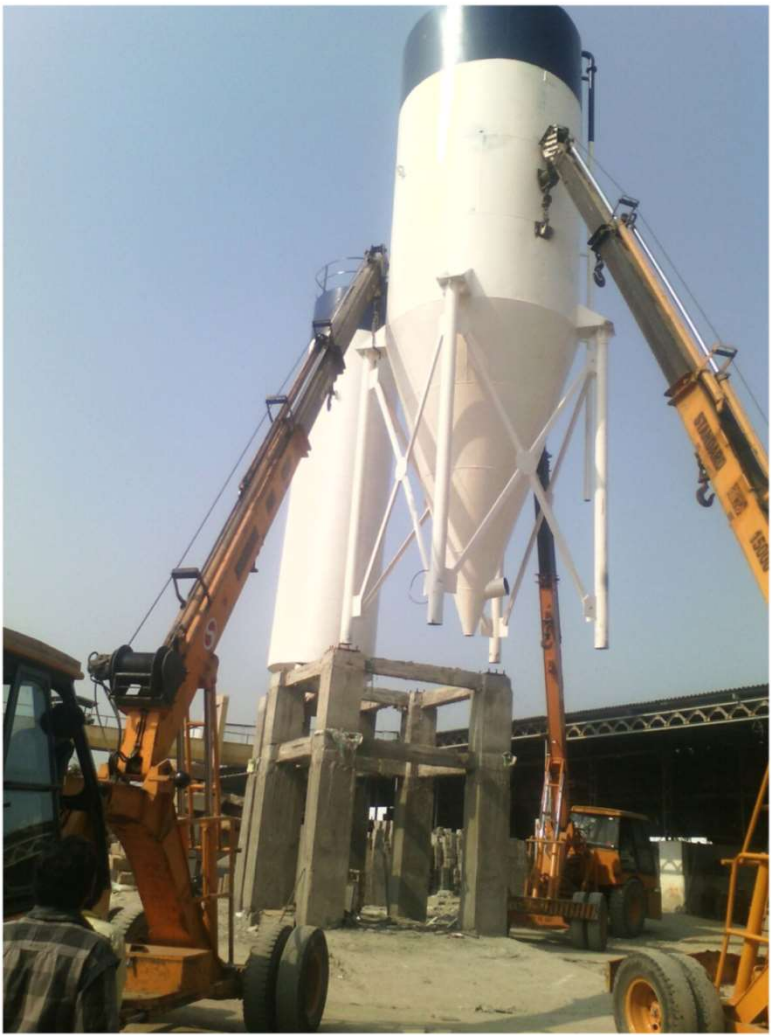
150 Kld Sedimentation Plant Florence Sand Stone, Bundi, Raj.
